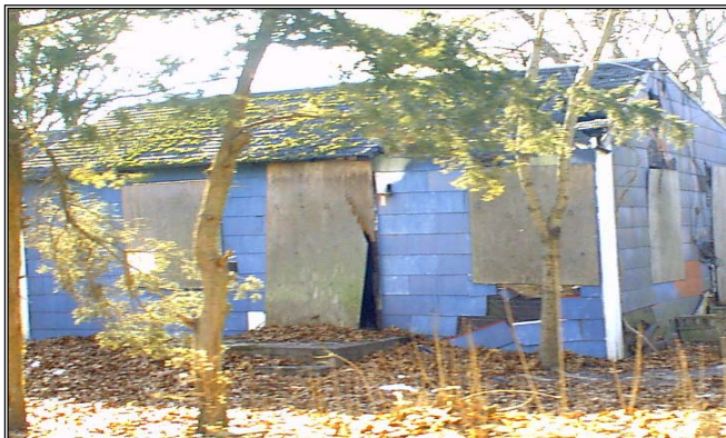
Severe housing blight on Old Quogue Road Riverside
